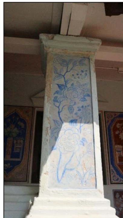
Figure 1.20: Unfinished restoration work of MLM Source: Field work
