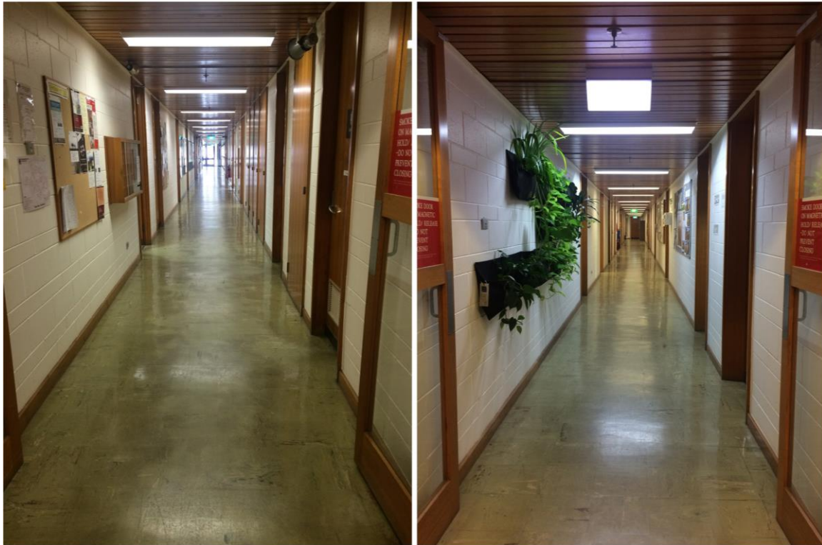
Figure 2: Images of north corridor (without iVGS) and south corridor (with iVGS). Picture taken from the building lobby.
