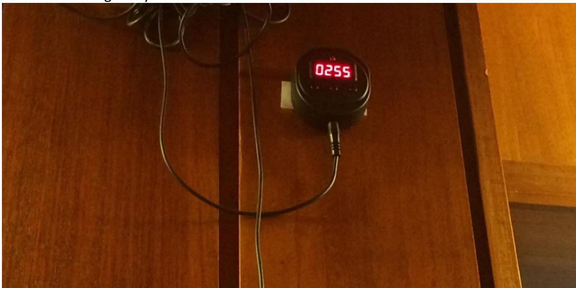
Figure 3: N287 Commercial Grade Doorway Beam unit installed in the north corridor.
