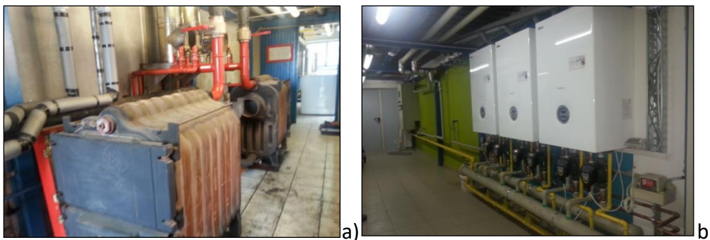
Figure 3. a) Modernization of heating systems (old thermal power plant - b) New thermal power plant
